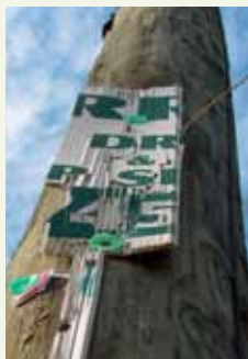
Staples, nails, and tacks used to hang signs pose dangers to Bluestem Electric's linemen.
