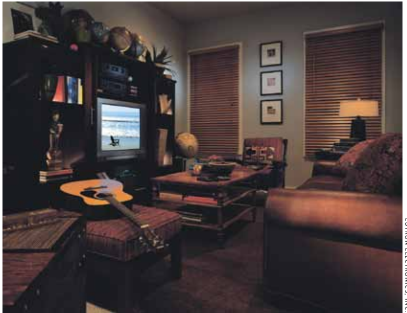
Central lighting control systems allow you to program special light levels for reading or watching movies.
