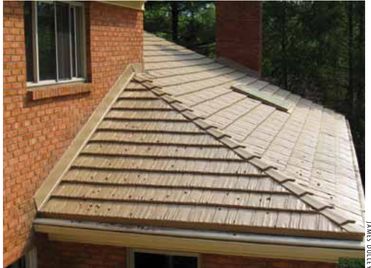
The completed metal roofing with new flashing and decorative hip trim over the seam makes an attractive presentation.
