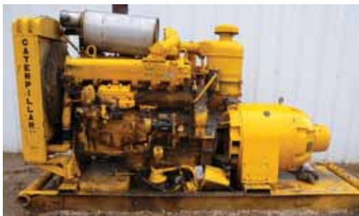
The diesel powered generator is believed to be a 1937 model. The purchaser is responsible for loading and hauling the generator.
