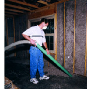
The excess is removed and the wall is typically ready for sheet rock within 24 hours.
