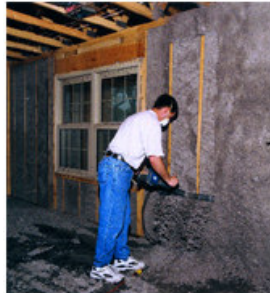
The product is blown into place, adhering to wood members, creating a monolithic seal.
